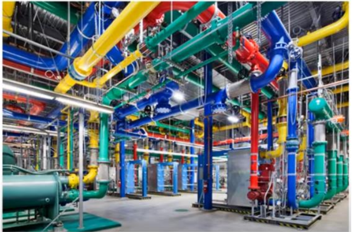
Image: Google Data Centre
